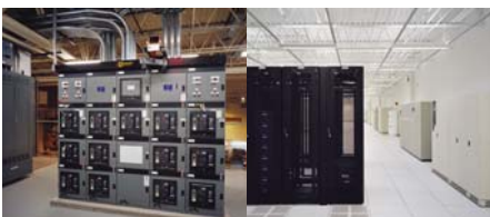
W.W. GRAINGER DISASTER RECOVERY CENTER Kansas City, Missouri Provided N+1 Backup Capability
