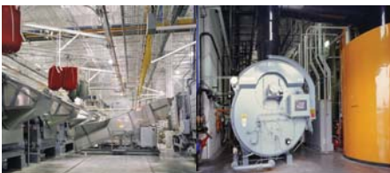
ARAMARK UNIFORM SERVICES Chicago, Illinois Utilized Energy Efficient Hot Water Recovery System
