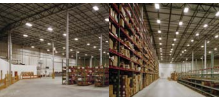
MEDLINE INDUSTRIES INC. Aberdeen, Maryland T5 Lighting Reduces Energy Costs
